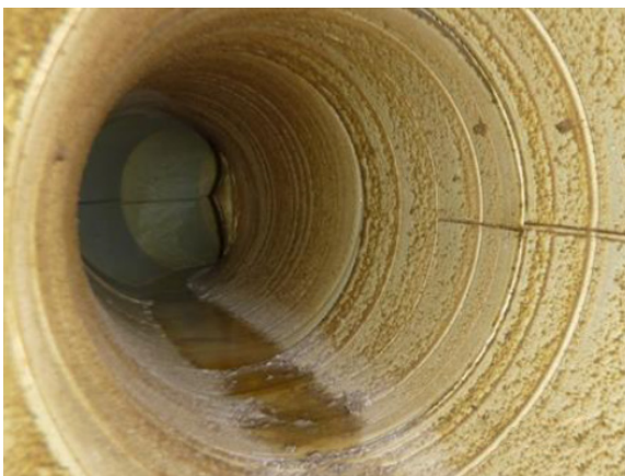
Without ozone cleaning system
